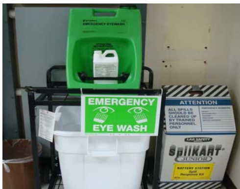
One of the many Emergency Eye Wash Stations installed at DOE Forrestral
